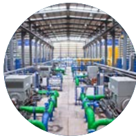
Utilities: Water, Heating & Telco
